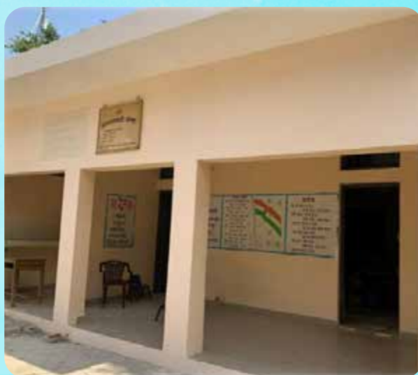
Painting work carried out at a government primary school in Naharpur, Manesar
